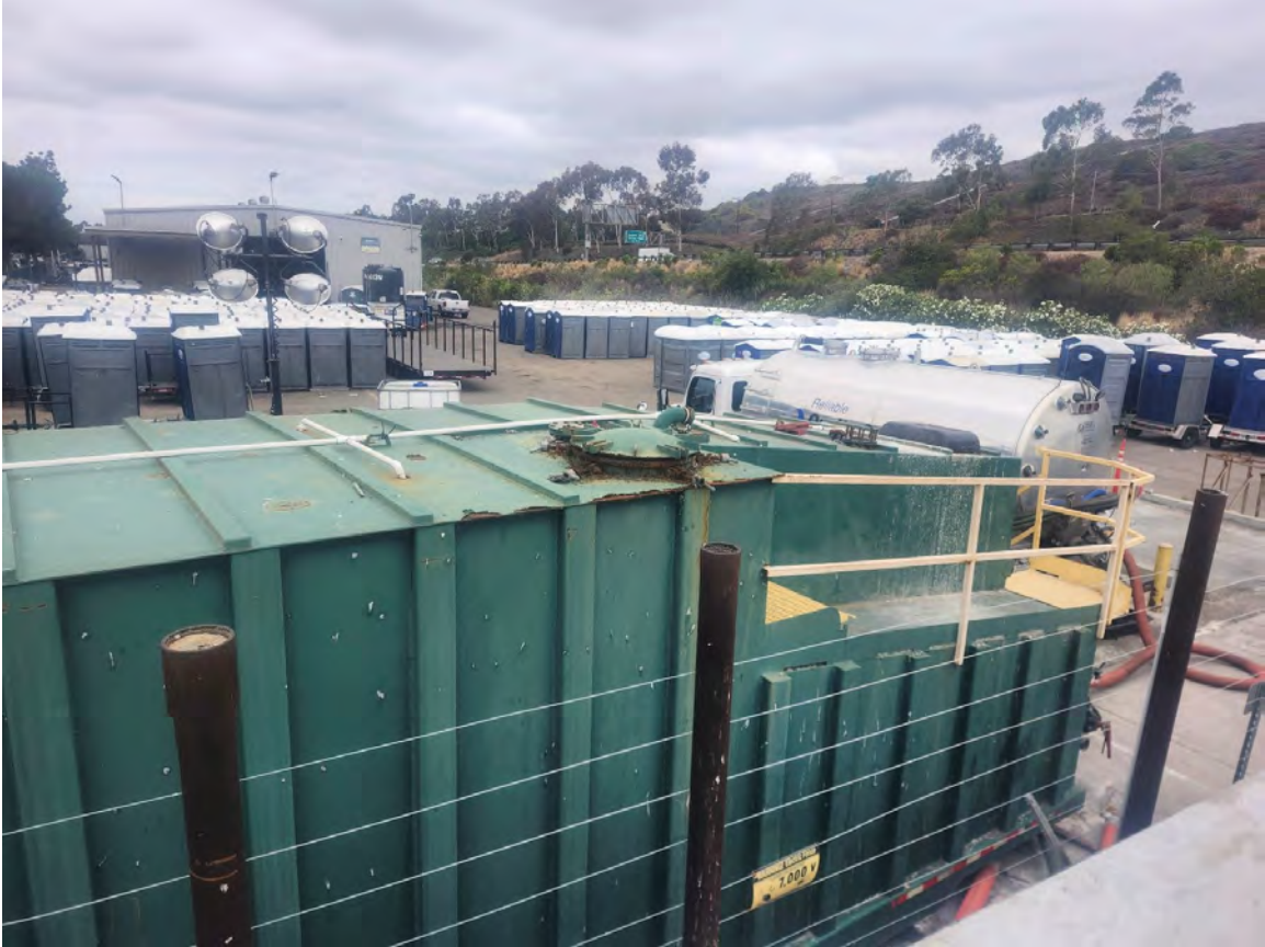
FIGURE 3. Top of the FRAC tank on an overcast day. The manway hatch and its collar are heavily rusted and a PVC vent line rises from the deck; a Reliable vacuum truck stands alongside. Corrosion at the tank's roof and vent — its pressure-relief points — is the subject of the separate FRAC-tank roof-vent corrosion analysis and bears on the safety of storing septage in this vessel. Photographed June 18, 2026 at 11:01 a.m.
