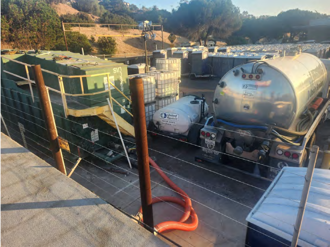
FIGURE 8. A stainless Onsite Services vacuum unit staged beside the FRAC tank, its placard reading “Capacity Waste – 4000” (Imperial Industries; California plate 95407F4). This is a dedicated 4,000-gallon septage hauler — a single, non-split tank with no cleaner compartment. CHART ONE lists only one 4,000-gallon non-split hauler on United Rentals’ 15-truck permit (line 12, plate 3533049), and its plate does not match this unit’s; whether this is that permitted truck or a separately registered unit cannot be confirmed from the photograph (see the discussion above). A coiled suction hose lies at the base of the tank. Photographed July 12, 2026 at 7:20 p.m.
