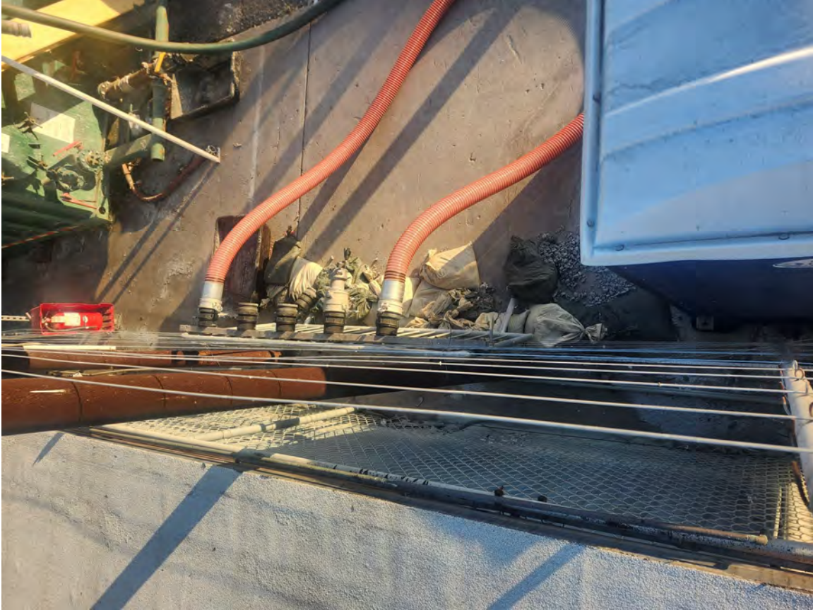
FIGURE 7. A fixed discharge manifold at the base of the FRAC tank — a row of cam-lock couplings for as many as five hoses, with two discharge lines connected and sandbags packed around the fittings. The sandbags are telling. Required secondary containment for septage is impermeable by rule: a sealed or lined base and berm sized to hold 110% of the vessel's volume, so that no leak reaches soil or storm drains (federal SPCC / 40 CFR 264.175 and the SDAPCD/DEHQ containment standard both require containment "sufficiently impervious" to hold the liquid). Sandbags are a permeable, temporary spill-diversion material — liquid weeps through and around them rather than being contained — so their presence at these fittings indicates seepage that is not being properly contained. This is permanent transfer infrastructure, not an occasional connection, and it raises a direct question for the record: the County DEHQ inspected this site on July 8, 2026 — the day before this photograph — and reported no violations and "no evidence of improper wastewater disposal" along the yard; how was an uncontained, sandbagged septage-transfer point not among the conditions that inspection documented? Photographed July 9, 2026 at 7:18 p.m.
