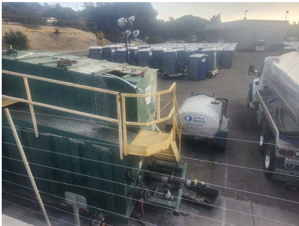
Fig. 17-7 — “20260717_184620.jpg” (≈ 6:46 p.m.). The green FRAC tank (asset SV3-3889-L) with the transfer plumbing and containment tray at its base along the boundary; staining down the vessel; the bulk hauler (plate 95407F4) at right; a white-poly supply tank at center, appearing roughly half full of what may be cleaning solution.
