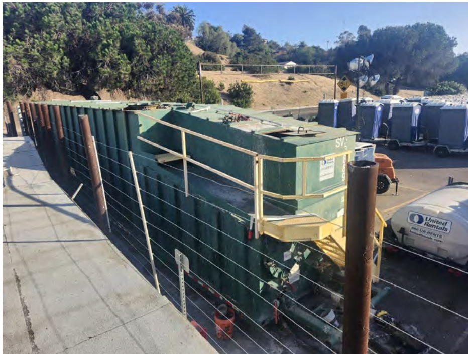
Fig. 2 — 20260716_181112.jpg (~6:11 p.m.). The green FRAC tank (United Rentals asset SV3-3889L) with the top hatch/manway standing open; access catwalk at right; staining down the vessel side. No attendant in view. Of note: with the warmer summer temperatures, the odor emanating from the open tank is overwhelming.
