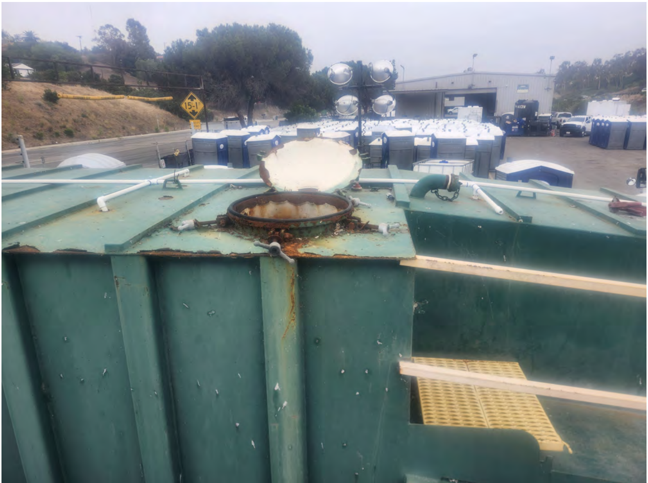
Image 1 — Roof hatch in the open position. Note the heavily rusted manway collar and rim, corroded swing bolts, and rust staining streaking down the shell below the opening; the flat roof panels and shell retain largely intact green coating. (4000 × 3000 px)
