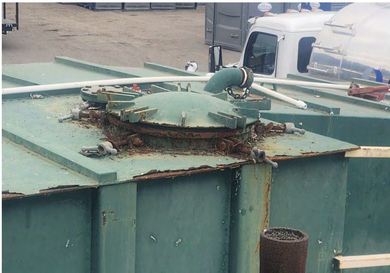
Image 2 — Roof hatch in the closed position. Flaking, laminar rust scale is concentrated at the lid-to-collar seam and surrounding hardware, while the broader coated surfaces remain sound. (1044 × 726 px)
