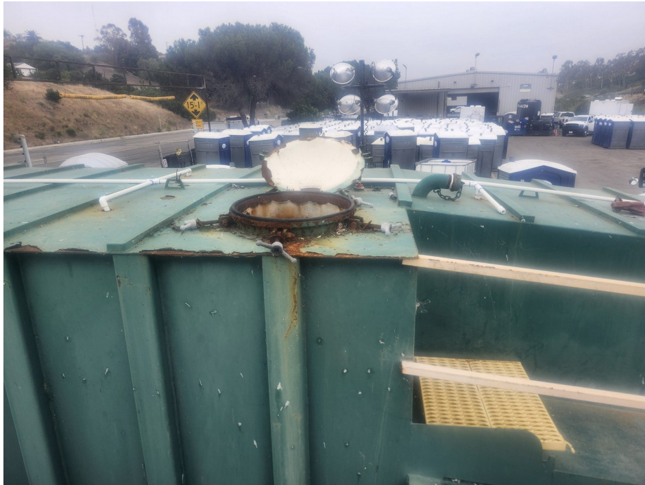
June 5, 2026, shows Mr. FRAC tank's roof hatch being open so that any of the sewer gases that accumulate from anaerobic digestion would escape into the atmosphere.
