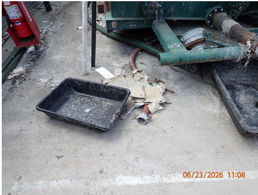
June 23, 2026 City of San Diego image taken by Inspector Daniel DeCurtins and produced in response to CPRA request no. 26-6563, showing rusted-out discharge piping and an open discharge hose with no secondary spill containment.
